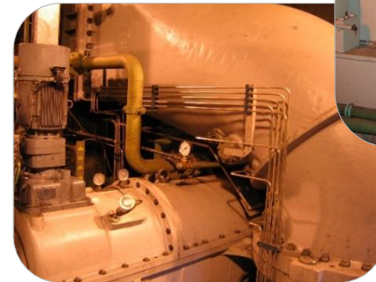
GHH Turbine + Generator 10MW
