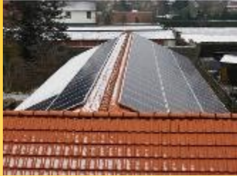
29 kWp Museum Langelsheim
